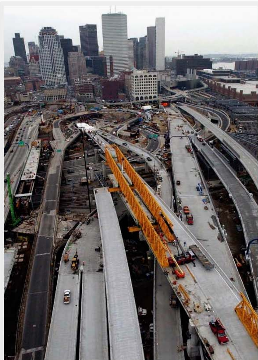
Construction of the Big Dig (Credit: David L. Ryan, "The Boston Globe")
